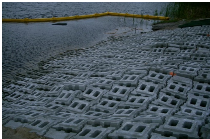
Figure 4. Subgrade Differential Settlement
