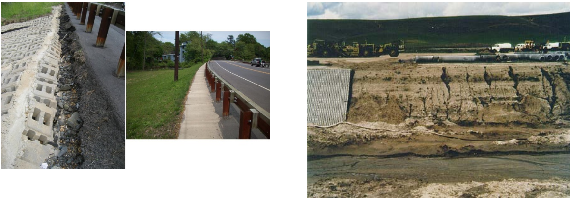
Figure 2. Examples of Installation Errors of ACB systems
