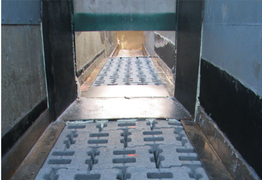
Figure 1 – Hydraulic gate installed 48.5 ft from top of slope to induce hydraulic jump Shoreblock SD 475 OCT
